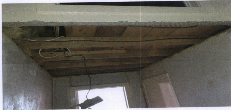
Picture 18: - Collapsed ceiling caused by burst water pipe and water damage.
