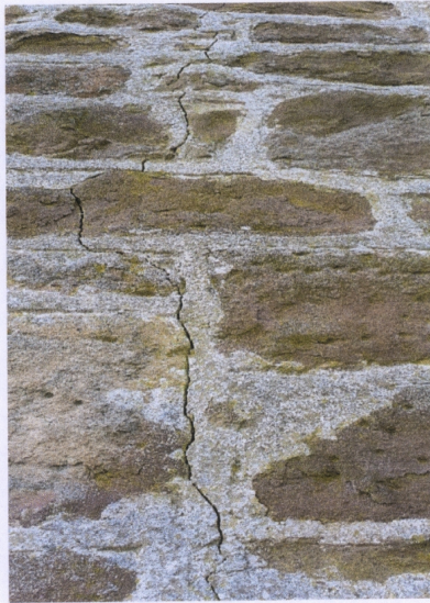
Picture 4: - Crack in gable wall
