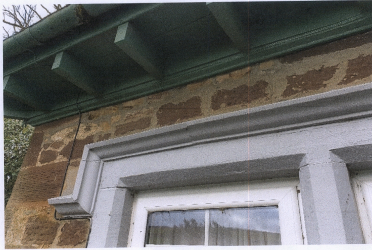
Picture 7: - Area above front left-hand side window where wall head has previously been raised
