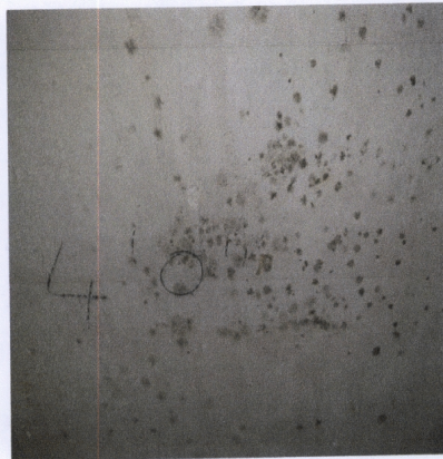
Picture 15: - Black mould throughout property
