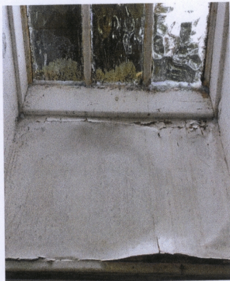
Picture 14: - Leaking kitchen roof
