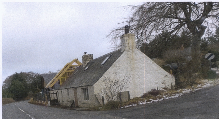
Picture 25: - Goldie's Mill, Note the height the roof is being raised to make the existing building and extension appropriate to each other in terms of SCALE . Also, a tree in close proximity to the building.
