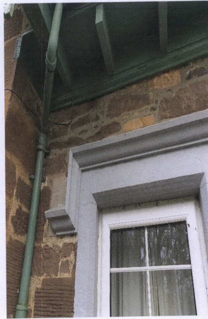
Picture 9: -Area above front right-hand side window where wall head has previously been raised.
